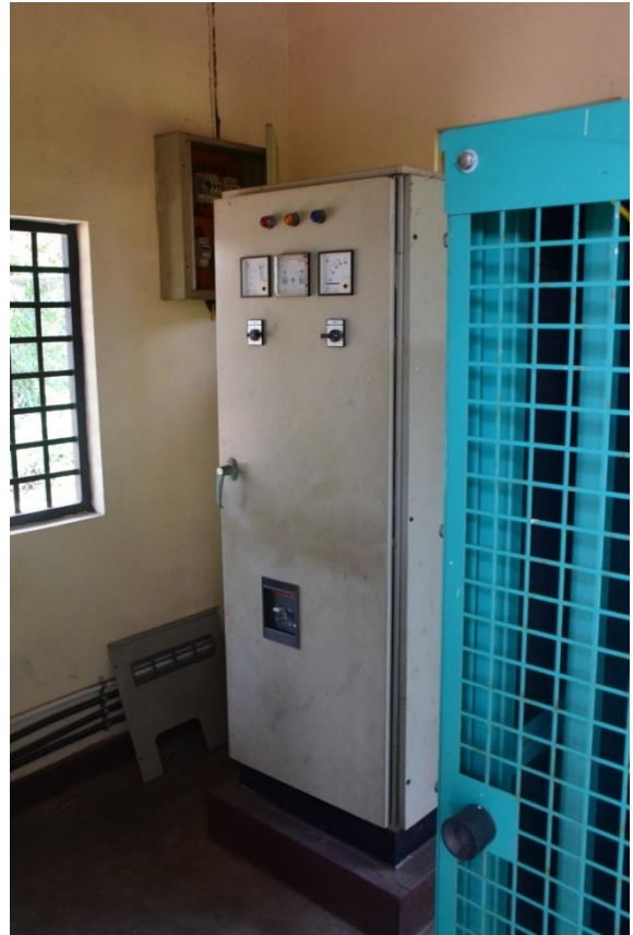
Generator- Kelaniya Holiday Resort
